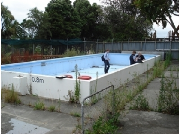
Figure 25: The Mt Pleasant School Pool being inspected for damage - 2013 post Earthquake (Source: Mt Pleasant School Archives, 2013)
